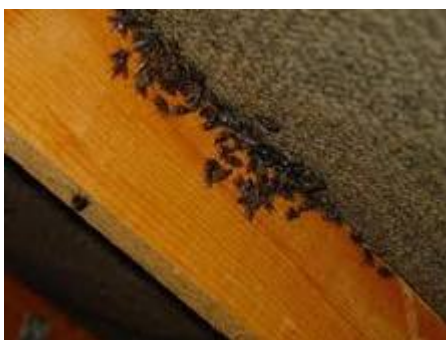
Cluster Flies in loft area
